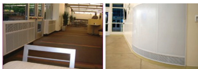
Fig. 8 : DV diffuser installed along the perimeter
